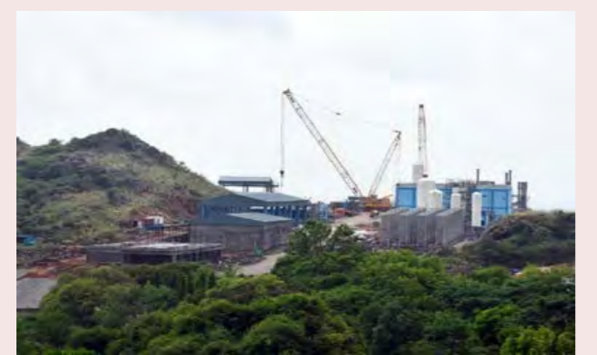
Integrated Cryogenic Engine and Stage Testing Facility
