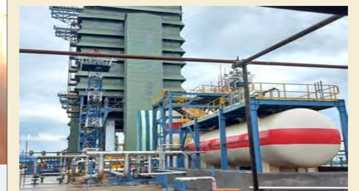
Cryogenic Fuel Storage Facility
