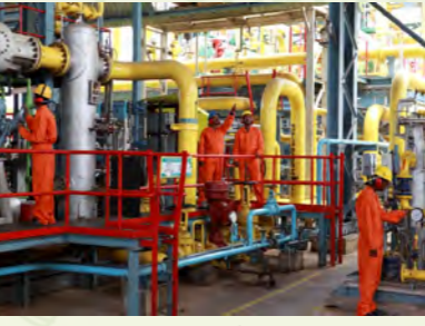
Gas Processing and Compression Facility ONGC, Rajahmundry, A.P
