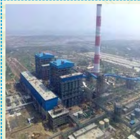
2x800 MW Sri Damodaram Sanjeevaiah Thermal Power Station, Krishnapatnam, Nellore (Dist.), A.P.
