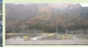
220KV Sub-Station in Nepal
