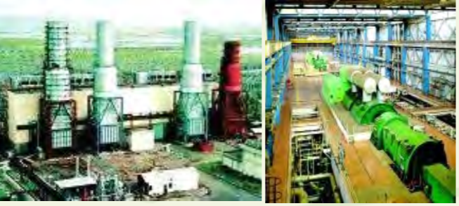
4 x 108 MW Power Plant, Uran, Mumbai, Maharashtra 500 MW Turbine Generator, NTPC Rihand, Uttar Pradesh
