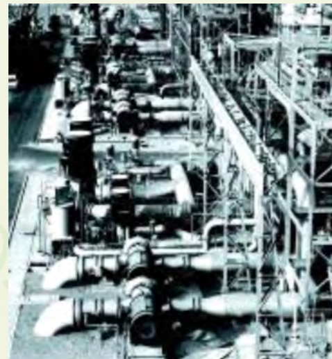
4 x 64 MW Power Station, Jeddah, Saudi Arabia
