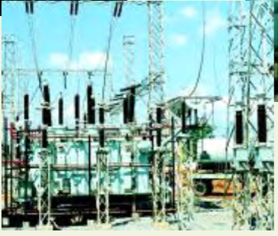
400 kV Switchyard, PGCIL, Orissa
