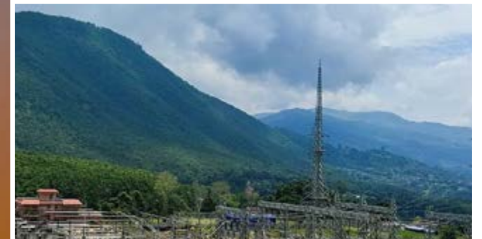
220 kV Kushma Substation Nepal
