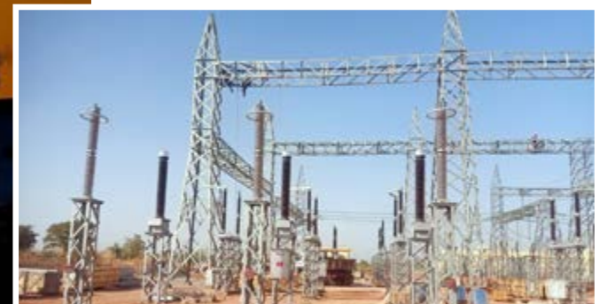
Sub-station project in Mali
