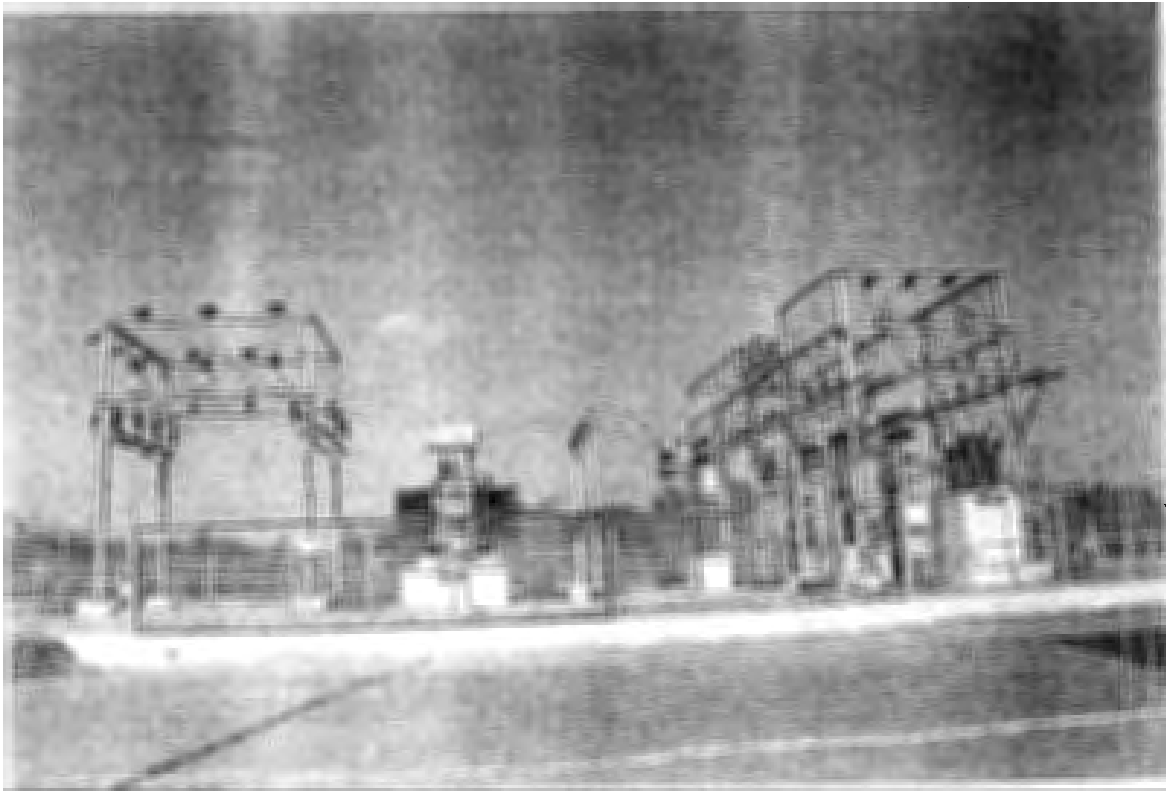
Construction of 33 KV/11 KV Sub-stations for OECF Funded Rural Electrification Programme at Warangal – Andhra Pradesh – Geesukonda Substation.
