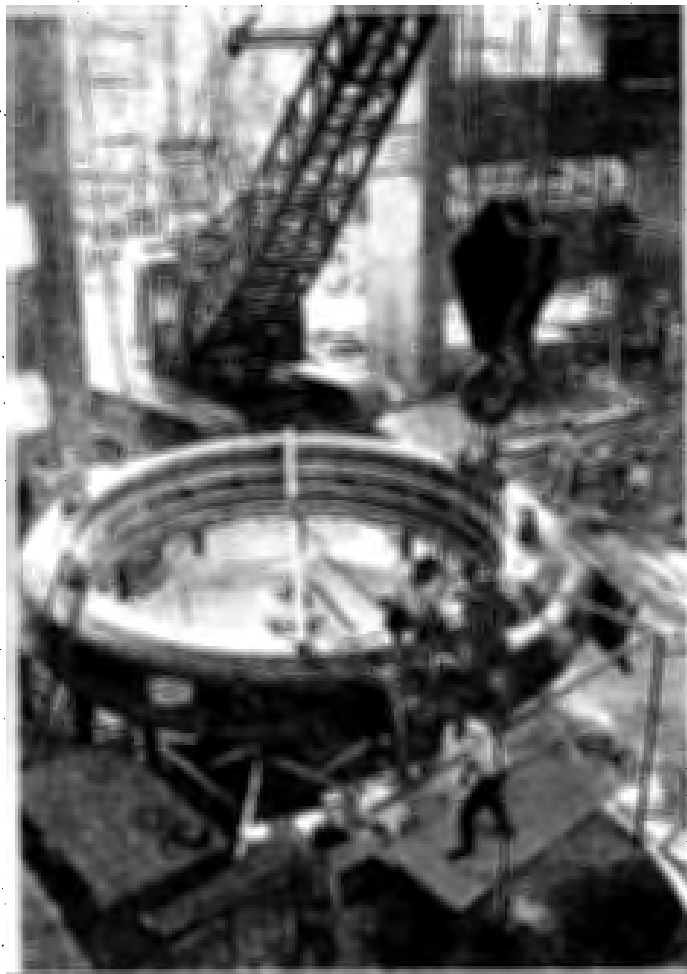
Welding of the Spiral Casing of 1x150 MW Pumped Storage Hydro Power Plant of Tata Electric Companies at Bhira, Maharashtra.
