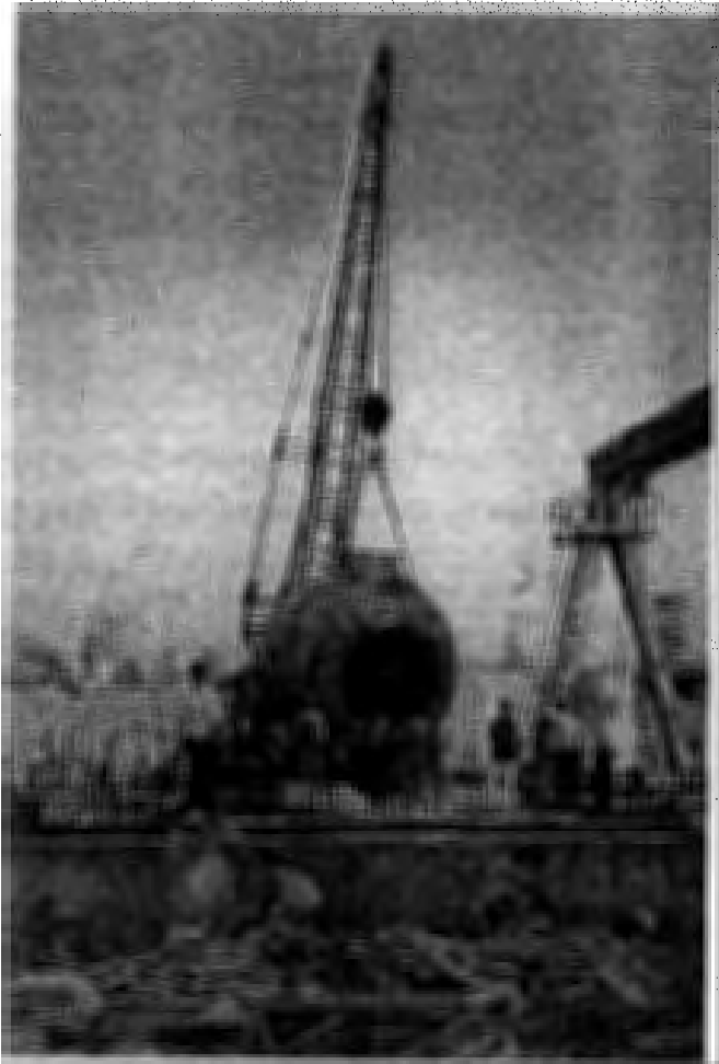
Positioning of Turbine Casing (33.7 M T) for 2 x 1.664 MW Sunsari Morang Mini Hydel Power Plant at Biratnagar, Nepal
