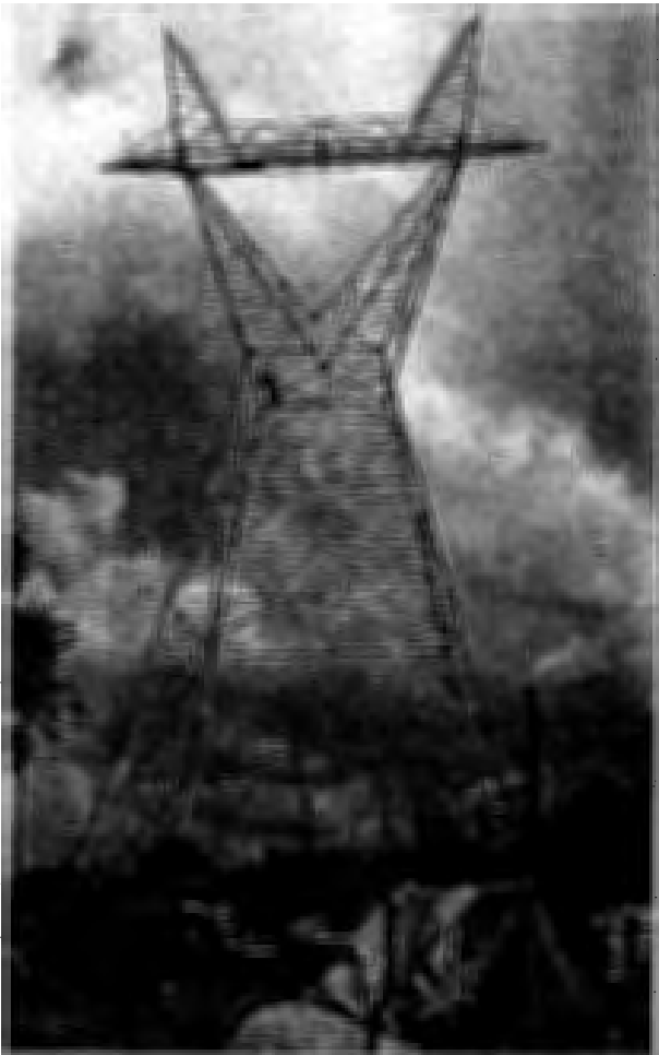
400 KV Double Circute Transmission Line Tower for Bihar State Electricity Board, Patratu, Bihar
