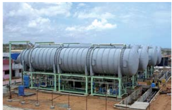
7680 m 3 /day Sea Water Desalination Plant, NPCIL, Kudankulam
