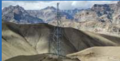
India's Highest Transmission Line (13,500 Feet)
